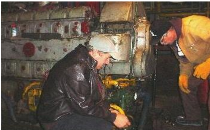
Bill Siebert and Larry LaChance working on the cooling for the aft ship's service generator.
