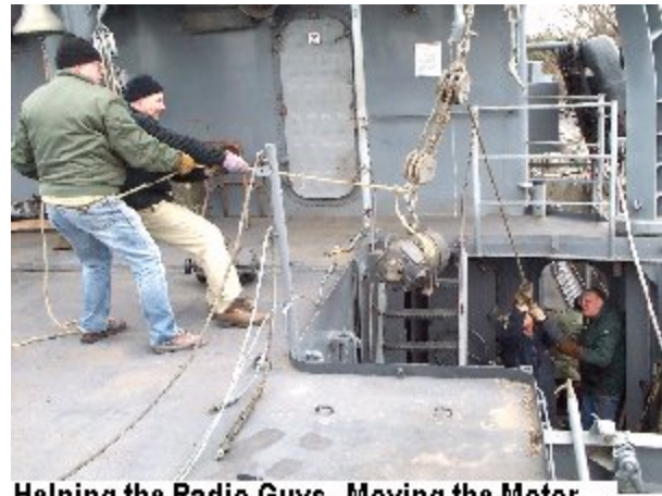
Helping the Radio Guys. Moving the Motor Generator Set into the Radio Room.
