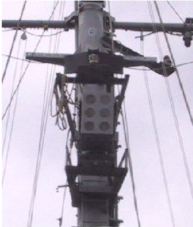
Closeup of Mast-Mounted Bullhorn Unit
