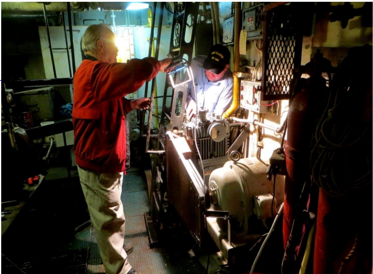
Karl and Mike installing the safety guard on the B-1 LP air compressor.
