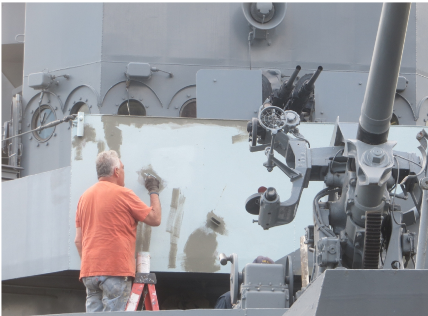
Anthony Amandola priming the pilothouse bulwark during the HUSE Assn. work week.
