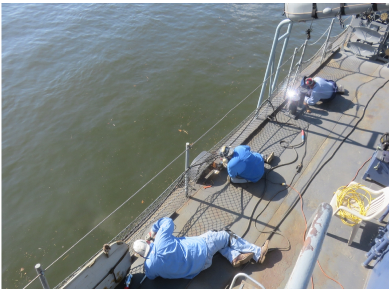
Three welders, no waiting. Ed's welder friends from the Limerick Nuclear Power Plant tackle our waterway problems.
