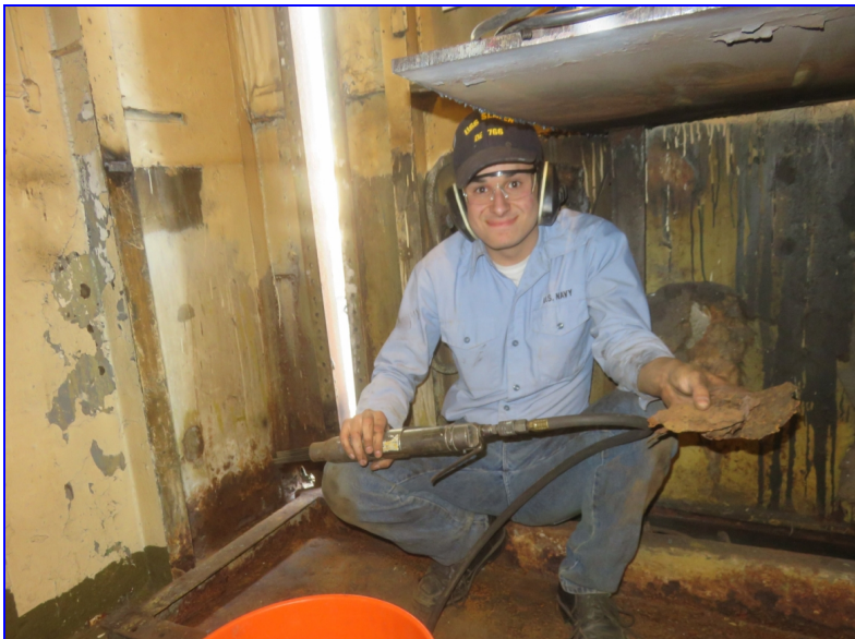
Thomas Scian cleaning and scaling where the machine shop work bench used to be.
