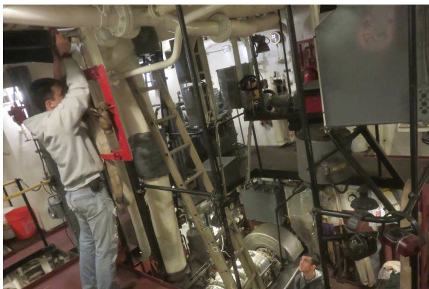
RPI Midshipmen Nick Grocki and Brian Beam helped drain down the firemain for the winter.
