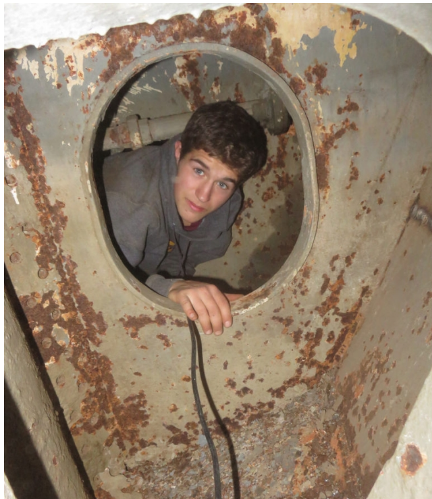
RPI Midshipman Parker Fields running electrical cable in the void below the steering gear compartment.
