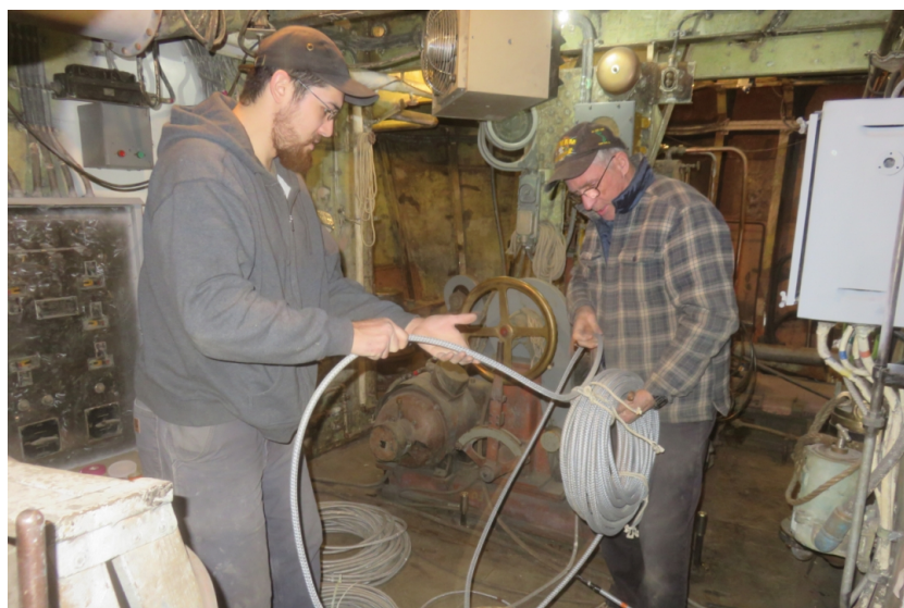
Ken Powers and Gary Sheedy running new power cables for the steering motors.
