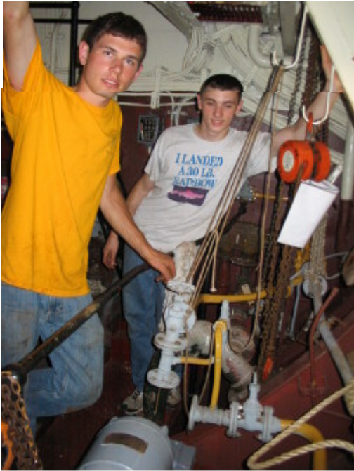
Engineering progress on the restoration of the motor lubricating pumps in B-4.
