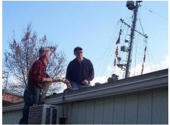
We spend all summer on the flying bridge fixing leaks over the director's office and now they want this roof fixed.
