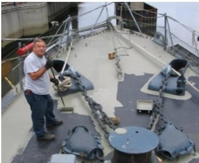
Before the dust settled Walt Stuart moved in and primed the deck.
