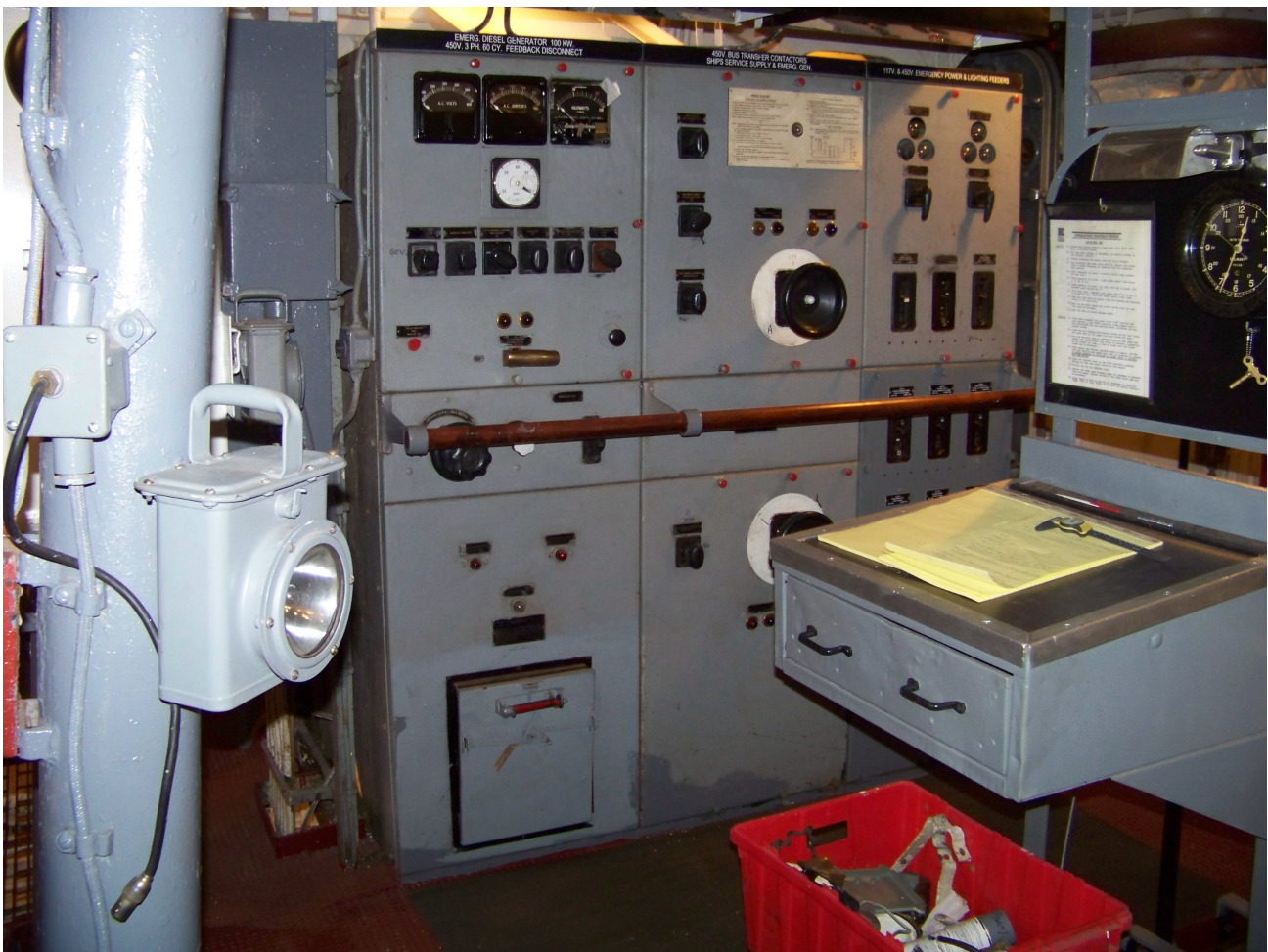
The emergency diesel switchboard.
