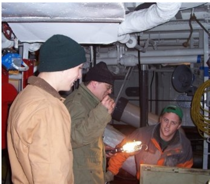
It was 20 degrees when Barry cleaned the switchboard.
