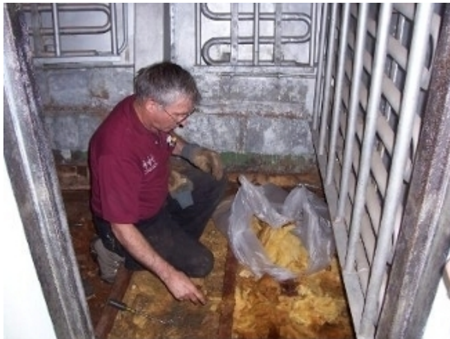
Gary Sheedy discovered a nightmare, water soaked fiberglass insulation below the false deck in the reefers. He is attacking the problem.
