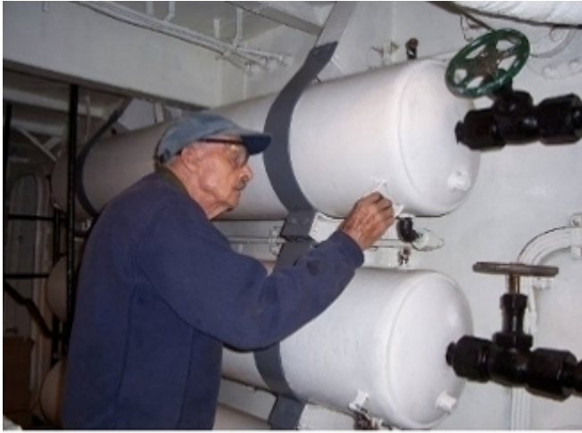
Rocky Rockwood restoring the starting air flasks in the aft engine room, B-3.
