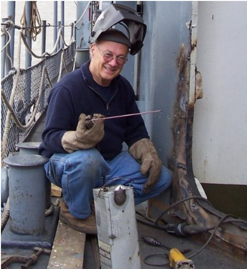
Dave Mardon has been spending most of his time cutting, welding & grinding at the new forward door.
