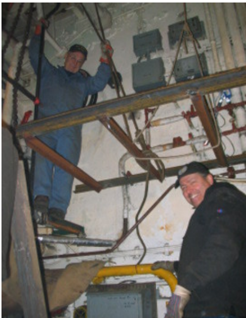
Don Miller and Bill Siebert repairing the catwalks in the aft diesel room.
