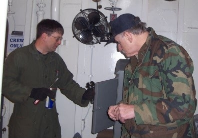
Barry Witte and Gordon Lattey prepping the power panel for the septic tank that will service the forward head.
