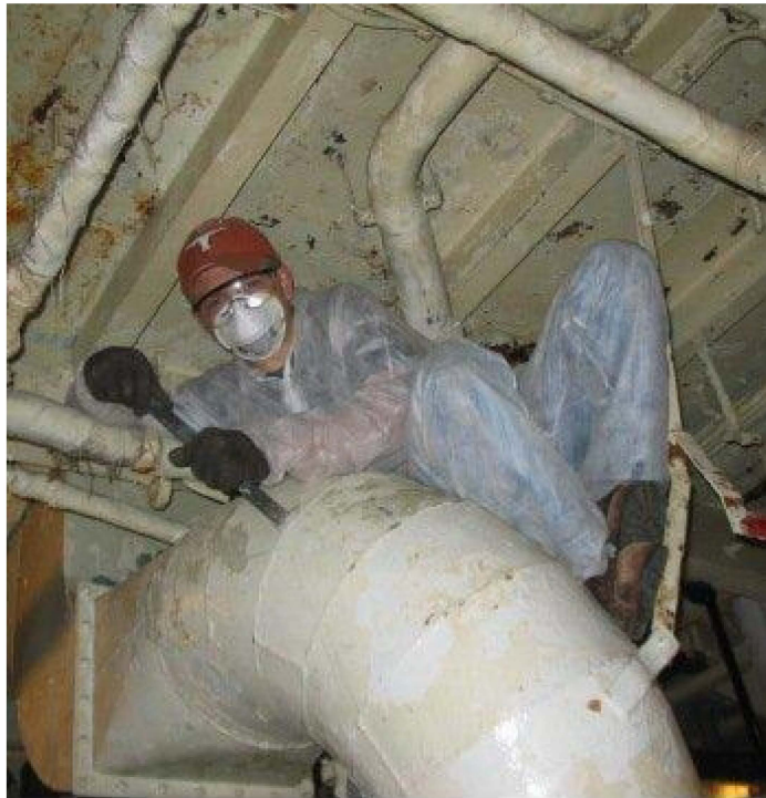
Josh Maurer hard at work chipping the top of a B4 fresh air duct while...
