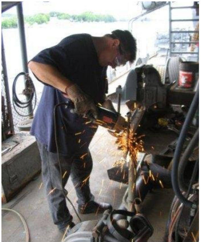
Bill Siebert grinding an angle iron to be used for engine room door bracing.
