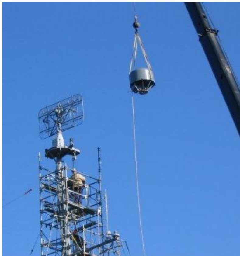
The SL radar dome is lifted on to it's new platform as Doug Tanner waits to bolt it in place.
