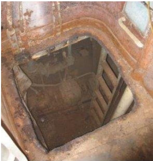
A rusted hatch and deck in the forward passageway will be replaced...
