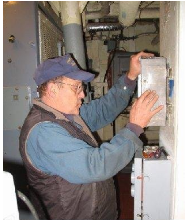
Gus Negus checks the fit on an engine-room electrical box.
