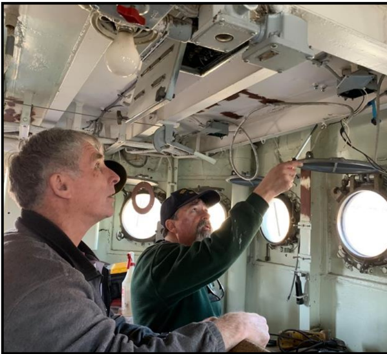
Gary and Steve work on the wiring to the windshield wipers in the Pilothouse.
