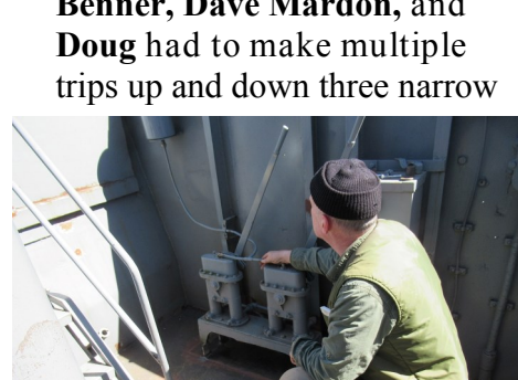
The installation of the depth charge release gear marked the completion of the flying bridge work.
