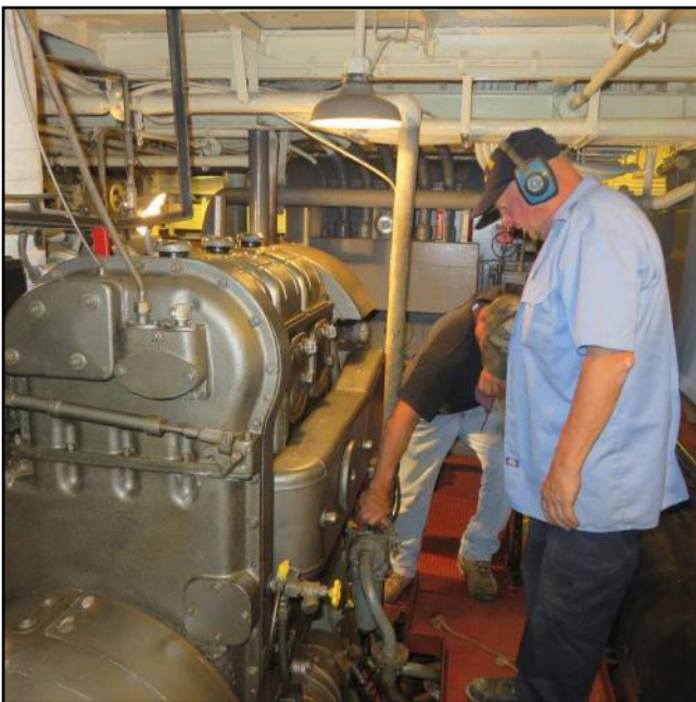
Mike starting the test run of the emergency diesel generator.
