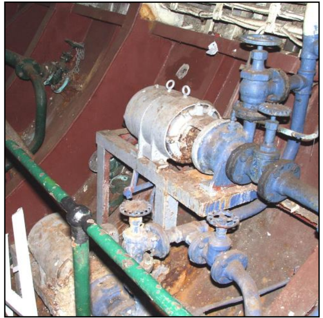
Fresh water pumps before restoration.
