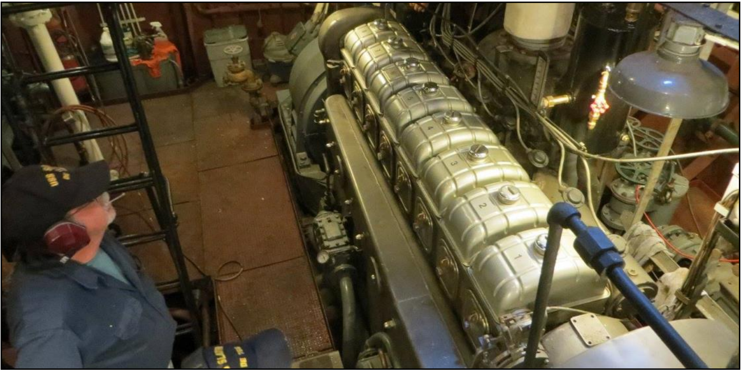
The engineers did a successful test run of the B-3 ship's service generator.
