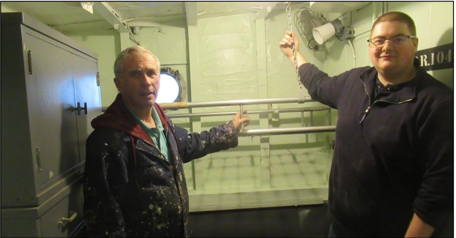
Gary and John install the first of the racks back into the Officer's Staterooms.
