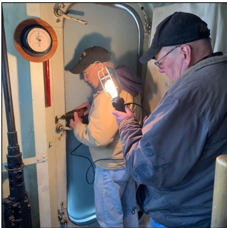
Dave and Warren finishing up installing this watertight door in the Pilot House.
