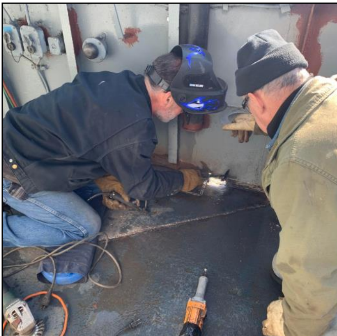
Together we can get this leak stopped.
