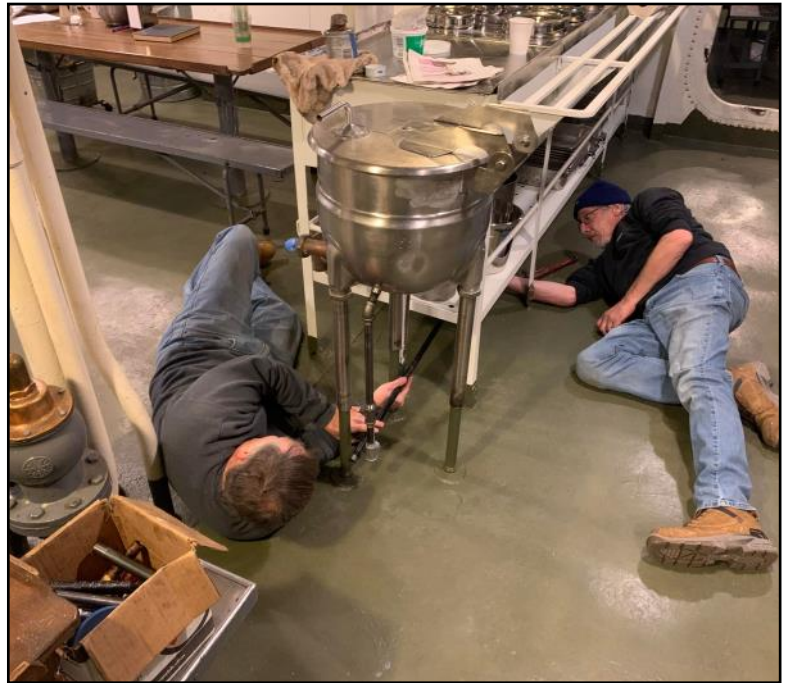
Barry and his crew put the finishing touches on the replica serving line.
