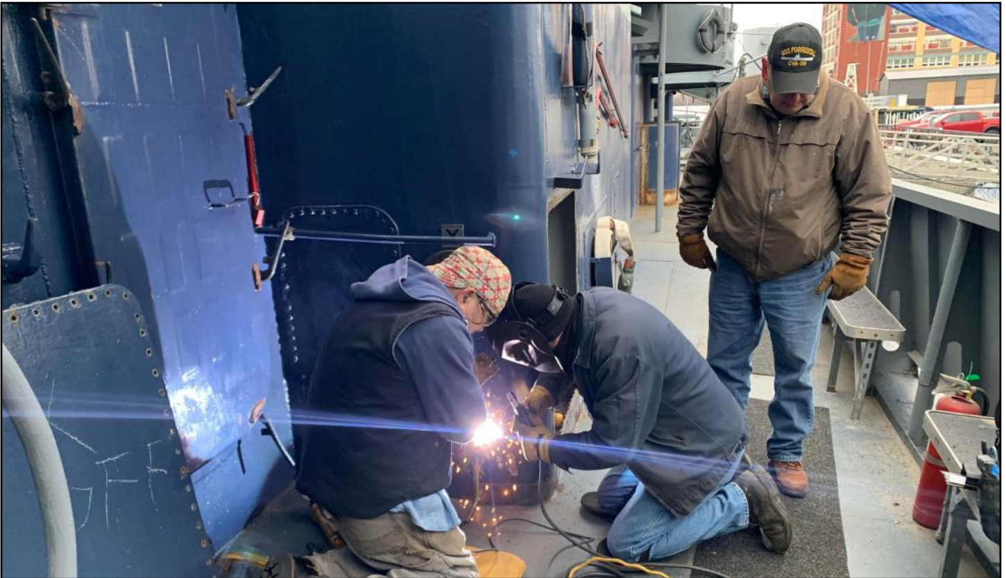
Doug and his shipfitters wrapped up repairs to the forward supply fan room.
