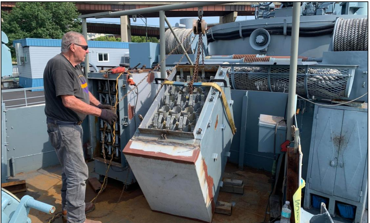
Danny Statile has involved all the shipfitters in the restoration of the Gun 33 ready service lockers.
