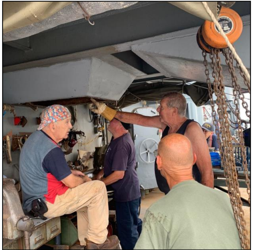
It takes the whole crew to fix the leaks in the deck above the work bench.
