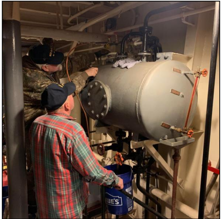
Jim and Mike performing maintenance on the emergency diesel generator day tank.
