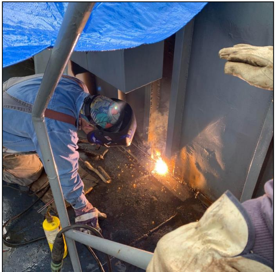
The rain doesn't stop Doug Tanner, as he repairs the flying bridge deck that was leaking into CIC.
