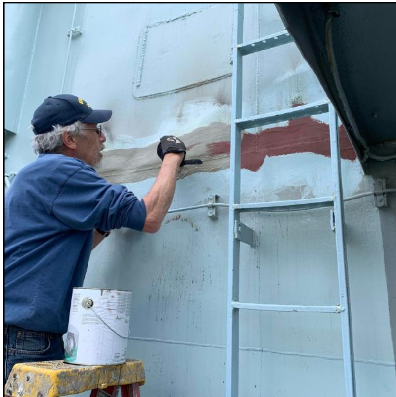
Bill Wetterau touches up the paint following the welding on the flying bridge.
